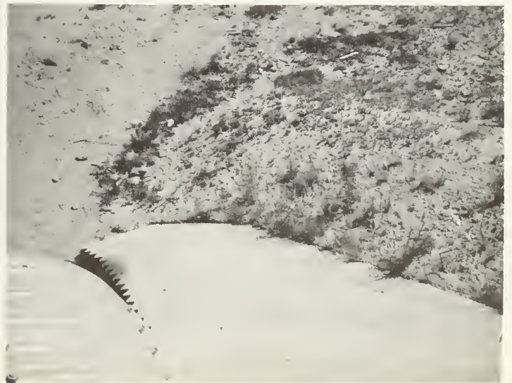
Closeup of cement facing; owner states cattle climb this area and slip and fall
